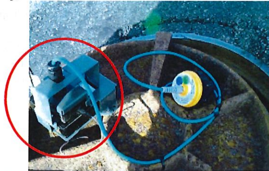
Bracket with E-Box and PowerPack on underside of manhole cover.
